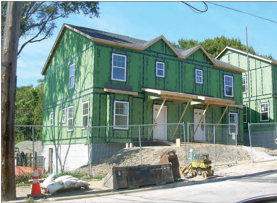
ABOVE: This 'Garfield Highlands' double house is in the 200 block of North Aiken Avenue. Photo by Rick Swartz.
